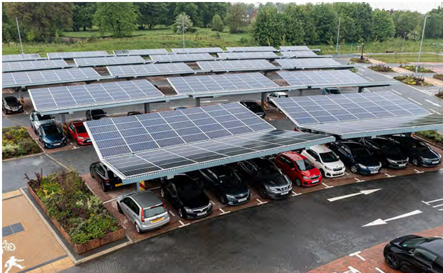
Solar panels, light weight shade structures, smart led lighting
