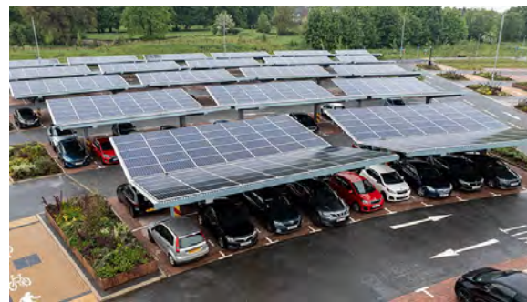
Renewable energy generation
